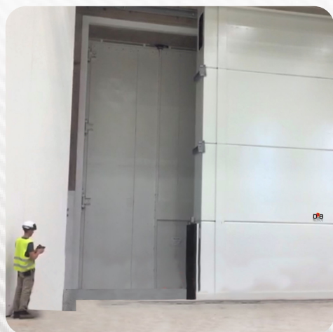
Porta blindata Rolls Royce 380 tonnellate - 12m*10m*1m
